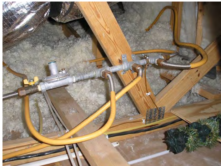
Manifold Installation with Grounding
