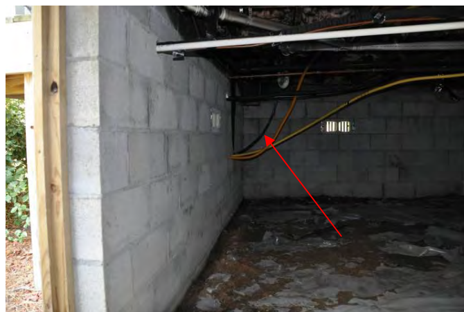
Location of CSST Hole Near the Wall
