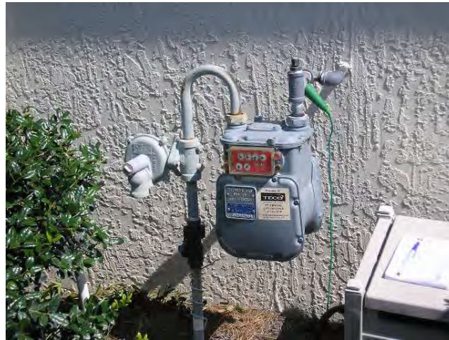
Impedance Test Point for Incoming Gas Line
