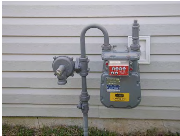
Gas Service Entry Point
