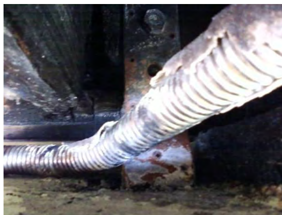
Location of the CSST Damage Near a Strap Connected through a Concrete Column to the House Basement
