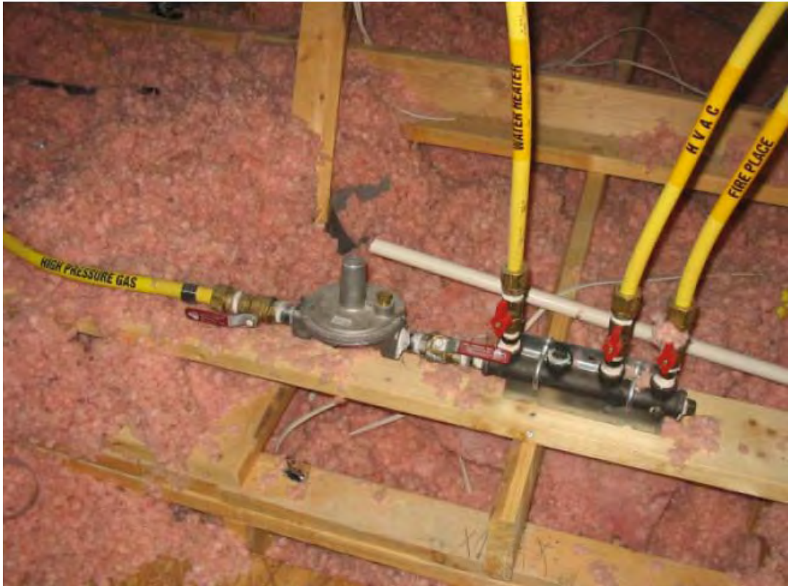
Attic CSST Installation without Visible Bonding
