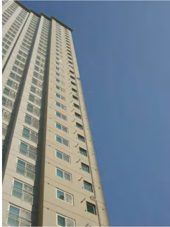
View of Gas Pipe on Right and Vents (One at Each Apartment)
