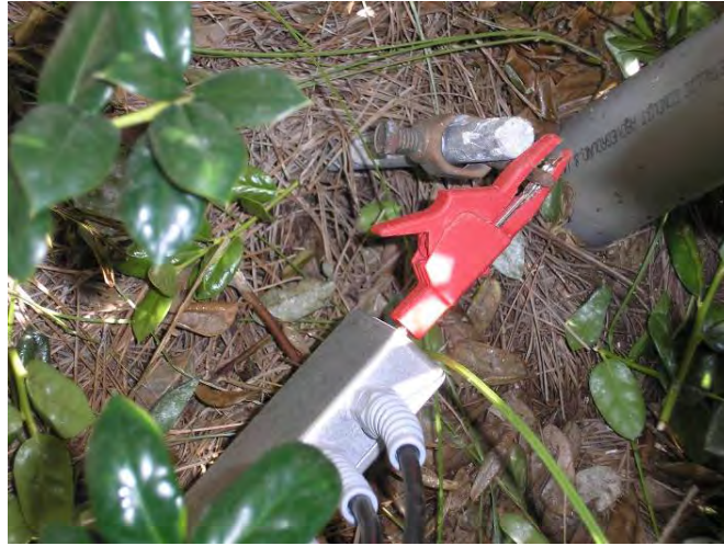
Grounding Electrode for Electrical Service and Manifold Ground Reference
