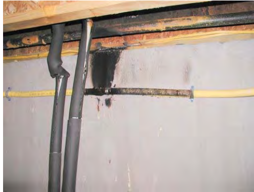
View of the Damaged CSST Near Two Vertical Plastic Pipes and Above CSST Electrical Cables, as well as a Metallic Pipe Run Horizontally
