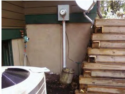
Electric and Gas Supply
