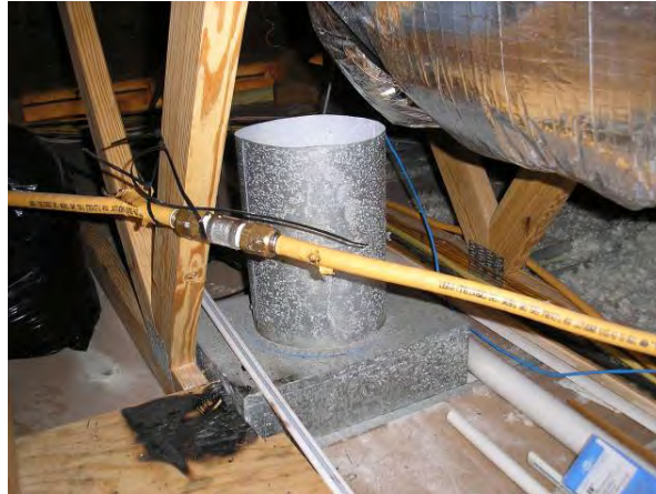
Place of Sparkover Between Metal Vent and CSST. (Note that CSST is now at distance from the initial position.)
