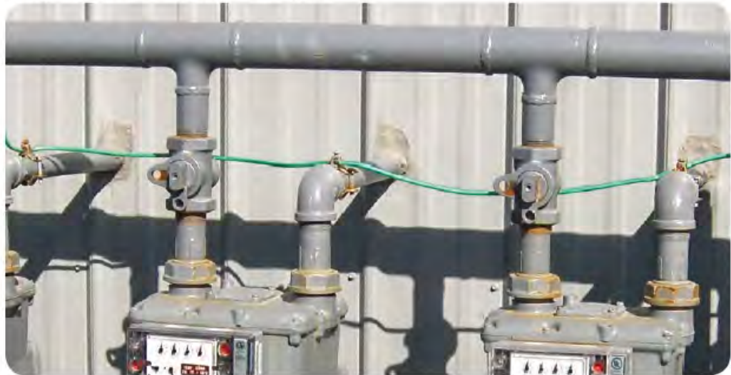
Acceptable CSST installation - example 2
